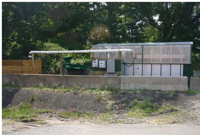
In vessel composting unit with biofilter at Joint Base Myer-Henderson Hall.
