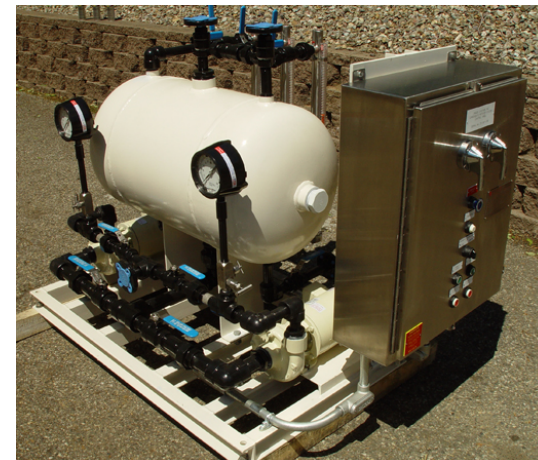
Condensate recovery system
